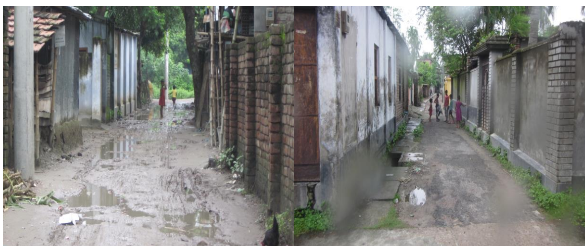
Pourashava road and drain with very badly damaged surface and displaying poor maintenance
